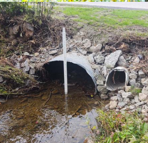
Culvert Before - severely restricting stream flow
