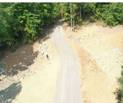
Figure 2: Creeley farm streambank protection and access road improvements just after final hydroseeding
