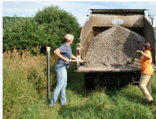
Amanda Barber and Kathy McGrath take shovelfuls of gravel from the town truck.
